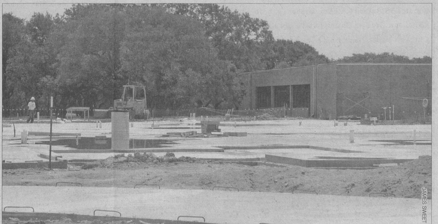
Much of the foundation has been poured at the new junior high construction site in Altair. The completion date for the project is one year away.
